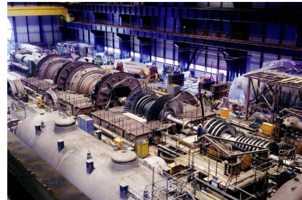
Electricity power plant
